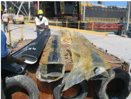
Retrowrap H Pile outer jacket with associated pre felted pre gelled filler blocks being loaded on work barge
