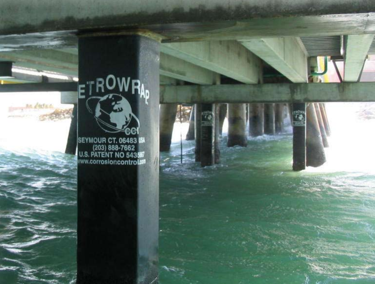
Vertical pile jacket showing outline (under fabric) of pile cap top seal seated at pile/ pile cap high stress interface
