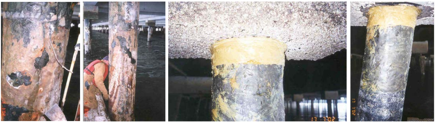
After damaged wrap removed, close up of blisters in existing epoxy visible.
