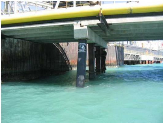
Full length outer jacket installed. Note Radius contour visible across pile flat face
