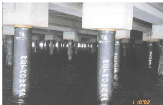
Impact and abrasion resistant Retrowrap HD retrofitted over piles where earlier installed wraps have been damaged.
