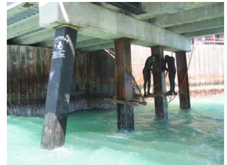
Temporary work platform attached to pile to permit upper pile cleaning and attachment of upper seal collar against pile cap
